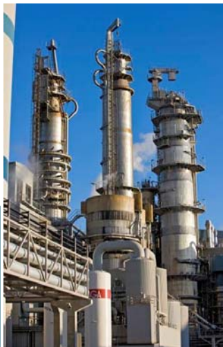
Continuous pulp digester 1, 2 and 3.
